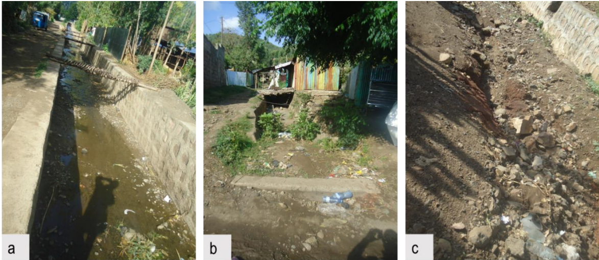
Figure 4:13 conditions of the existing drainage lines: good (a), moderate (b), and bad (c) Source: Field visits (2020)
