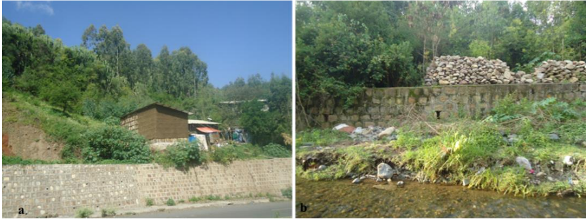
Figure 4:19 Retaining wall constructed to protect soil subsidence from mountainous areas (a) and river banks (b) Source: Field visit (2019) and computed by the author (2020)
