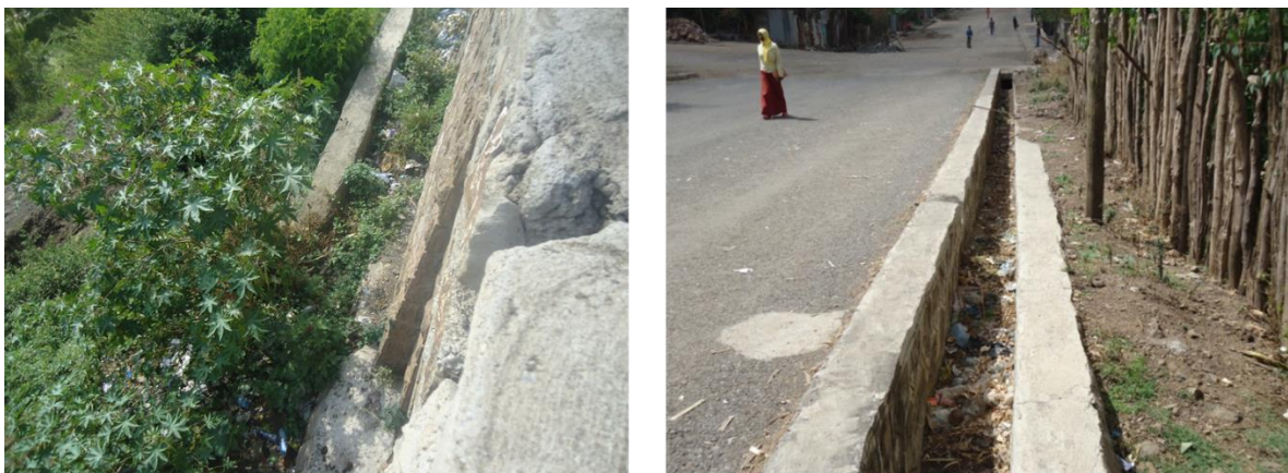
Figure 4:15 Open ditches filled with solid wastes Source: Computed by the author (2020)
