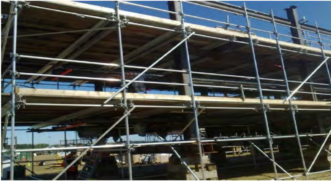
Figure 2.1 Tube and coupler scaffolding [4]
