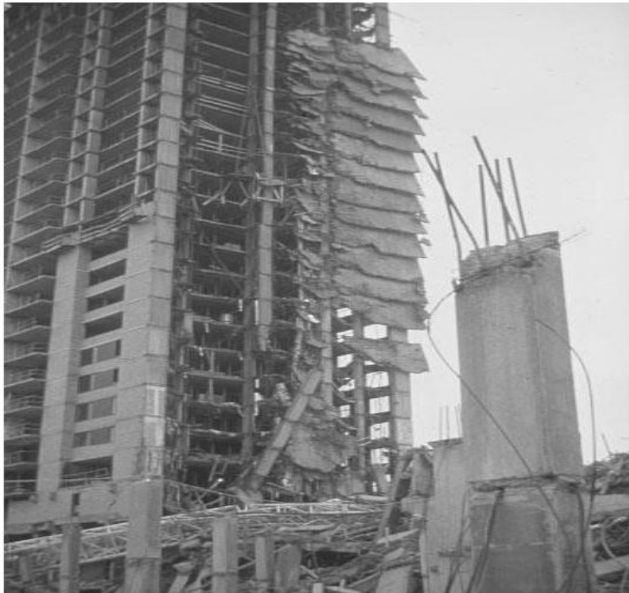
Figure 2.17 Progressive collapse of Skyline Apartments whilst under construction [53]
