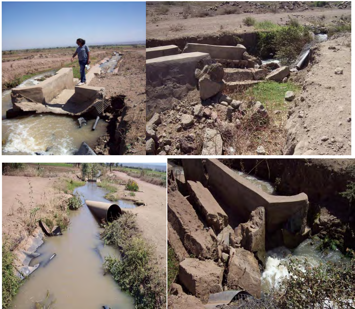
Figure 4.10 Structures that damaged by flood in Fentale irrigation project
