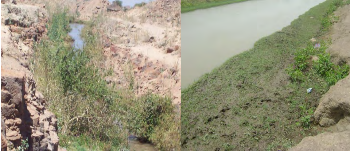
Figure 4.4 Silt up and weed growing along the canals
