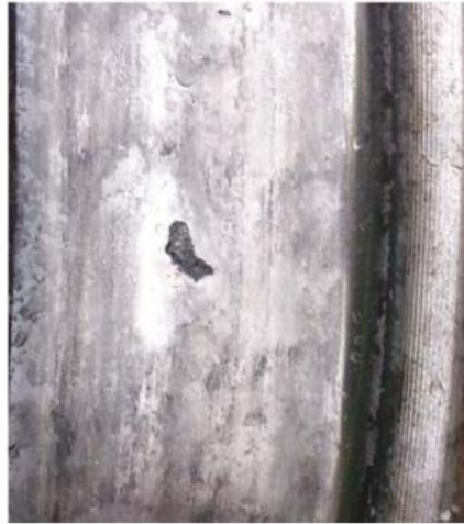
Figure 2.12: Damage under radial curving
