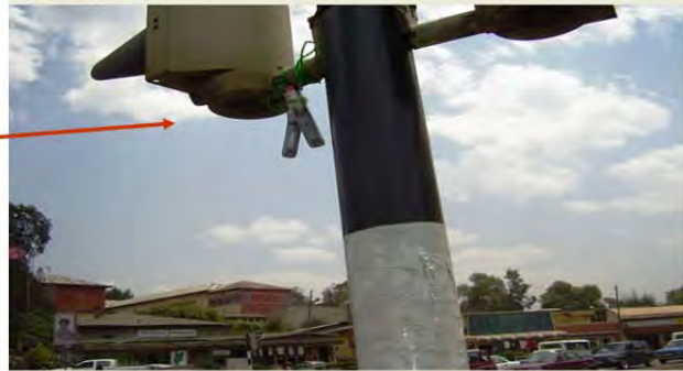
Figure 15: Field location of CO monitors on a traffic light stand, Addis Ababa, Ethiopia, April 2008
