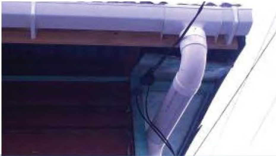
Figure 4: Typical PVC Guttering and Downpipe (Source: UNEP, 2009)
