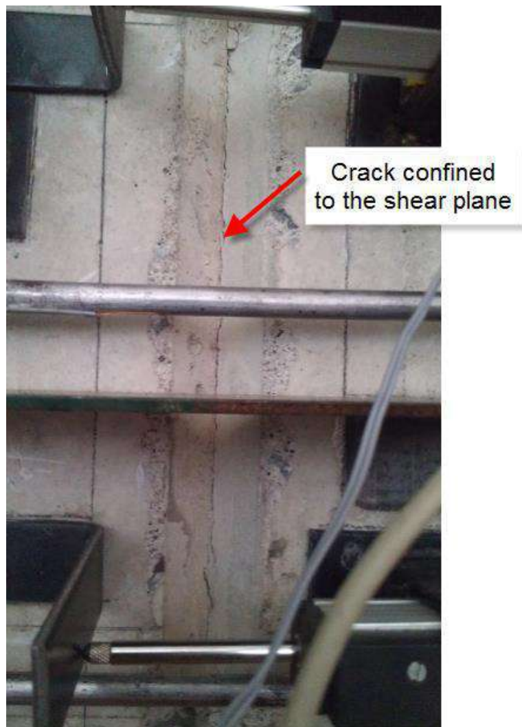
Figure.4. 16: Cracks formed in the first stage
