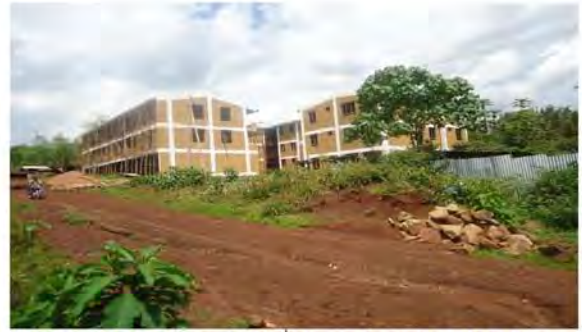
2006Ec only three blocks of condominium building at Mulu-wengel site, in a state of no site problem for massive development.
