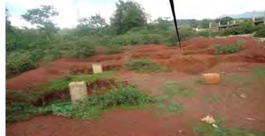
2007Ec Mituma site (industry & residence in plan proposal) 8 blocks condominium buildings situation & construction level, terminated even parts of footings not constructed, currently all reinforcement bars in the footing columns cut off & taken away.
