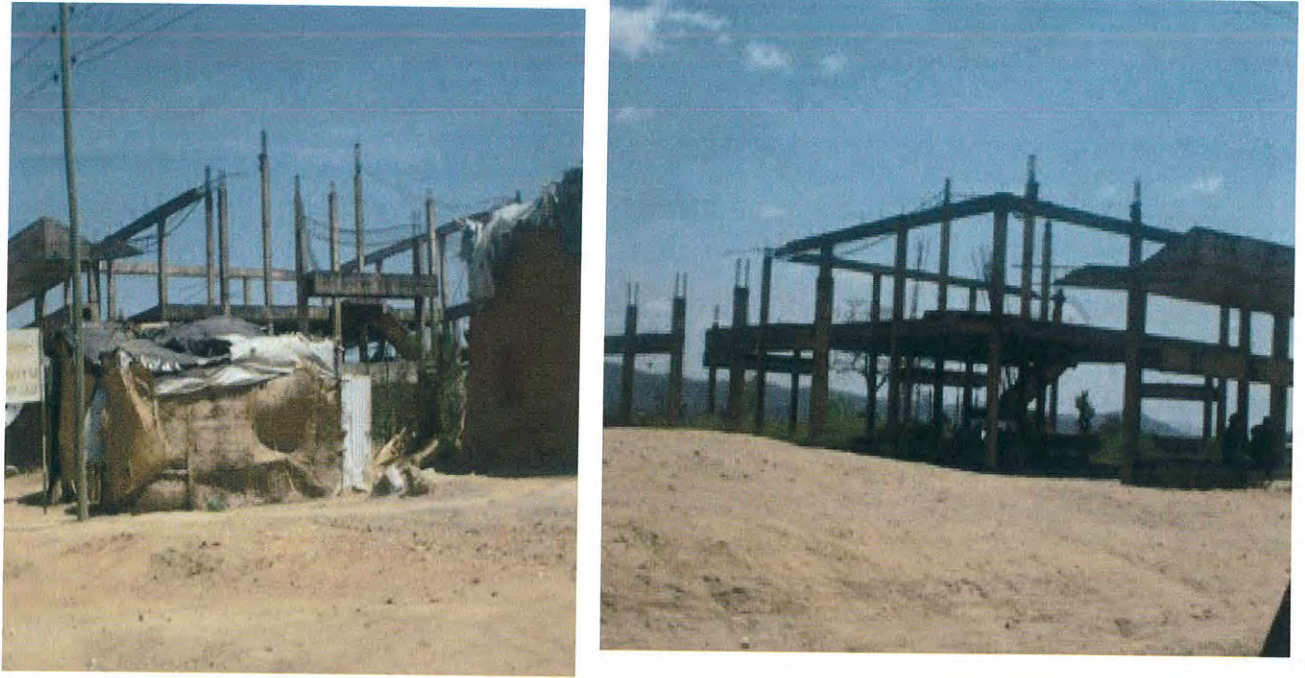
Figure 13. Incomplete constructions due to restriction by the local governments.
