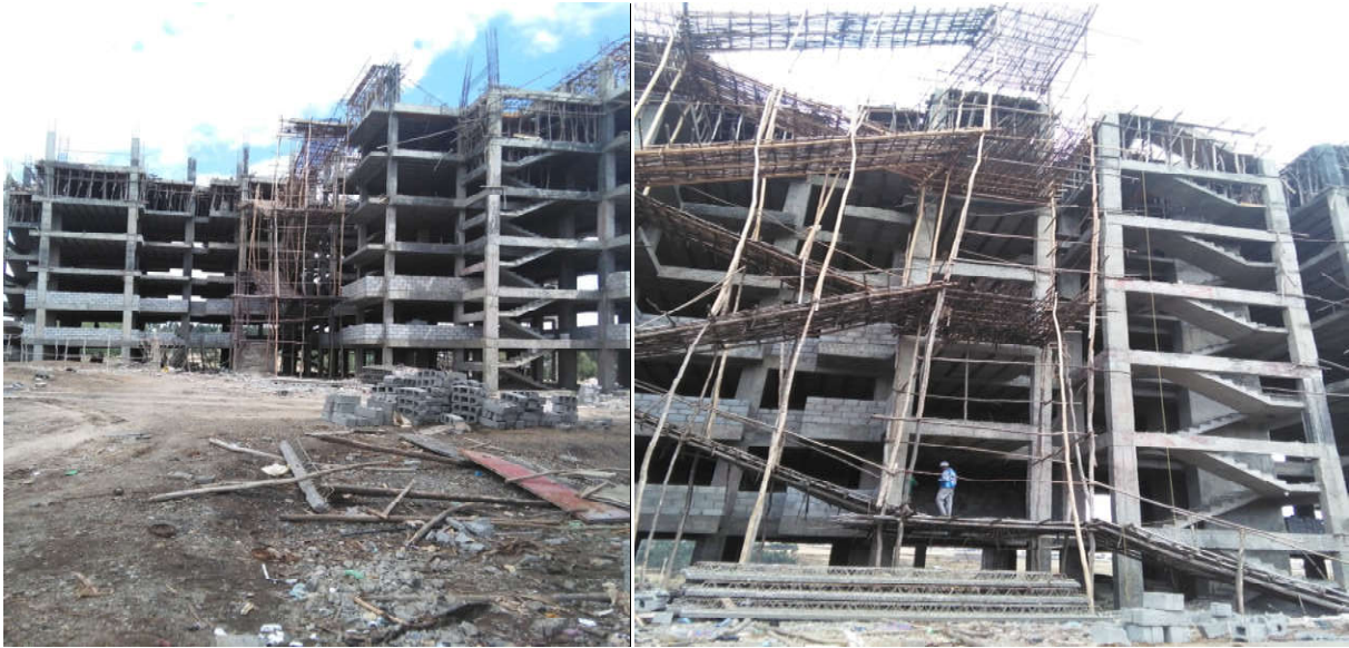
Figure 4.6 Partial view of Condominium Houses Buildings on Construction at Bole Arabssa Building Site; Source: Photo by the Researcher
