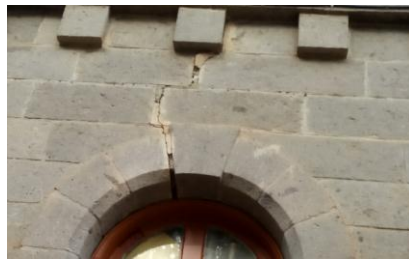
Figure 39 CRACK ON TOP OF THE ARCH OF WINDOW
