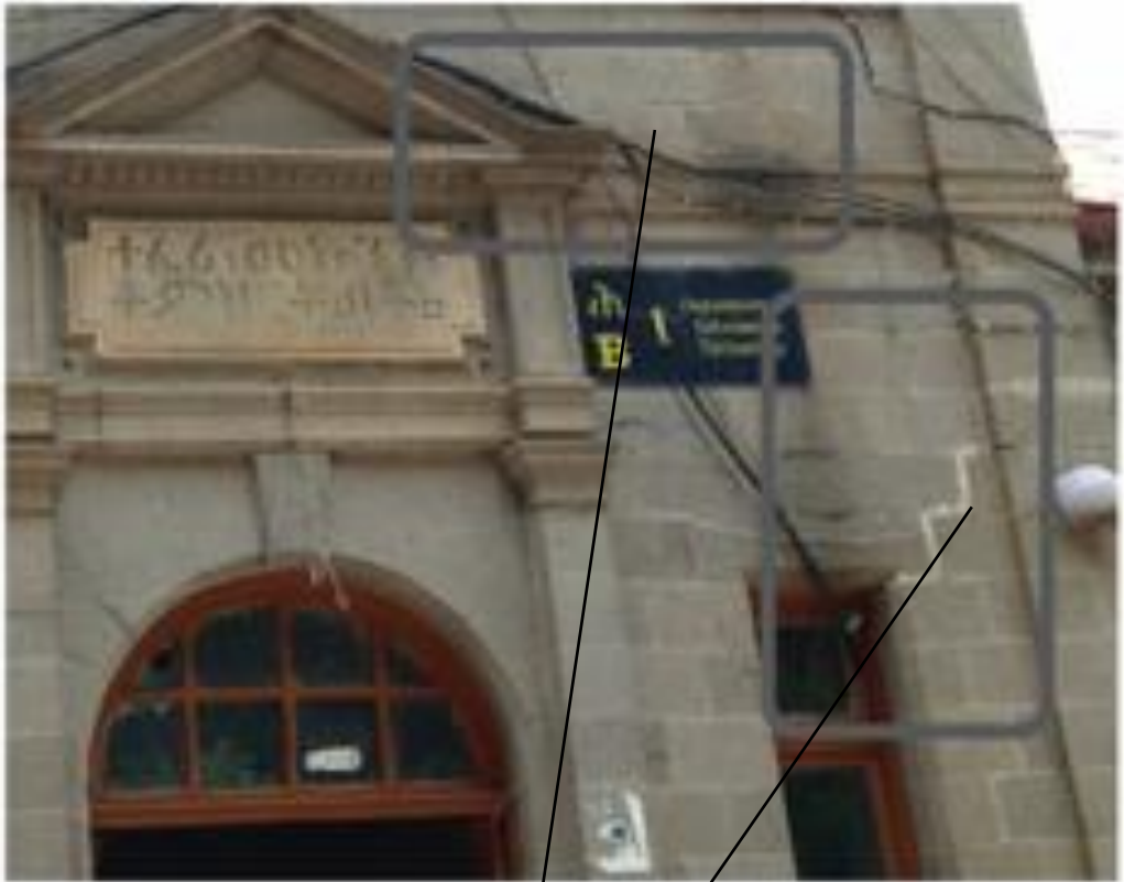
major crack on top of the window and improper mortar fill
