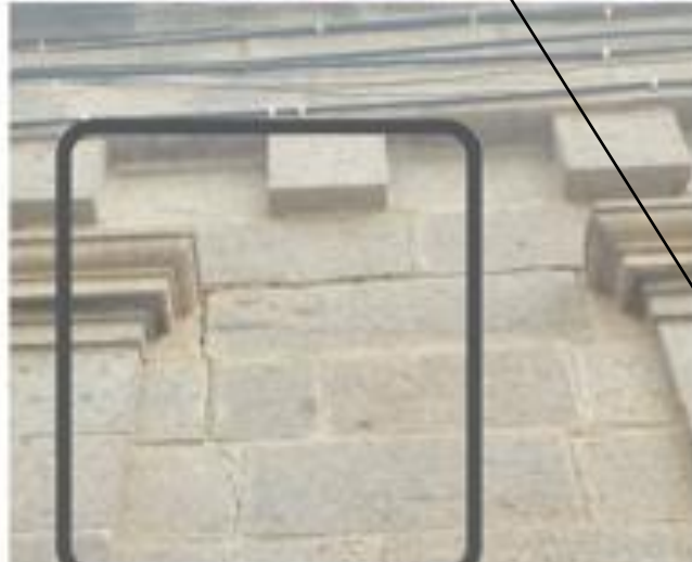
Location – front elevation right above the rectangular window
