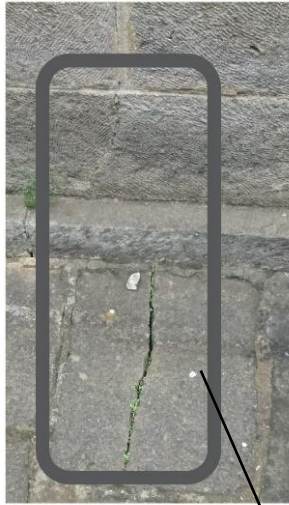
Location – front walkway crack
