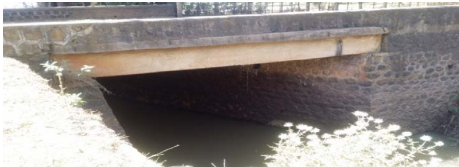
Figure 4.2 Improper site selections
