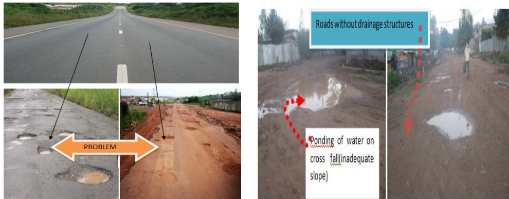
Figure1.2 Some deteriorated roads (lack of proper drainage)
