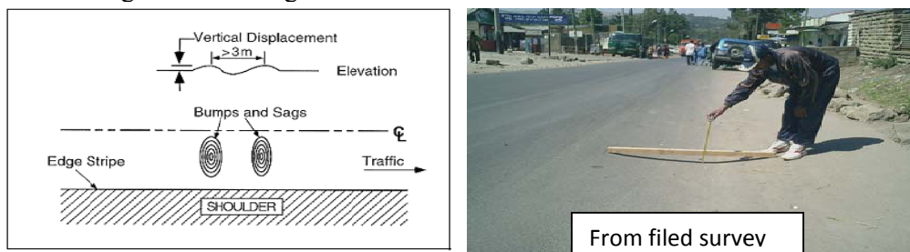
Figure 2.6 Bumps and sags from site survey & severity level as per(GTC, 1998)
