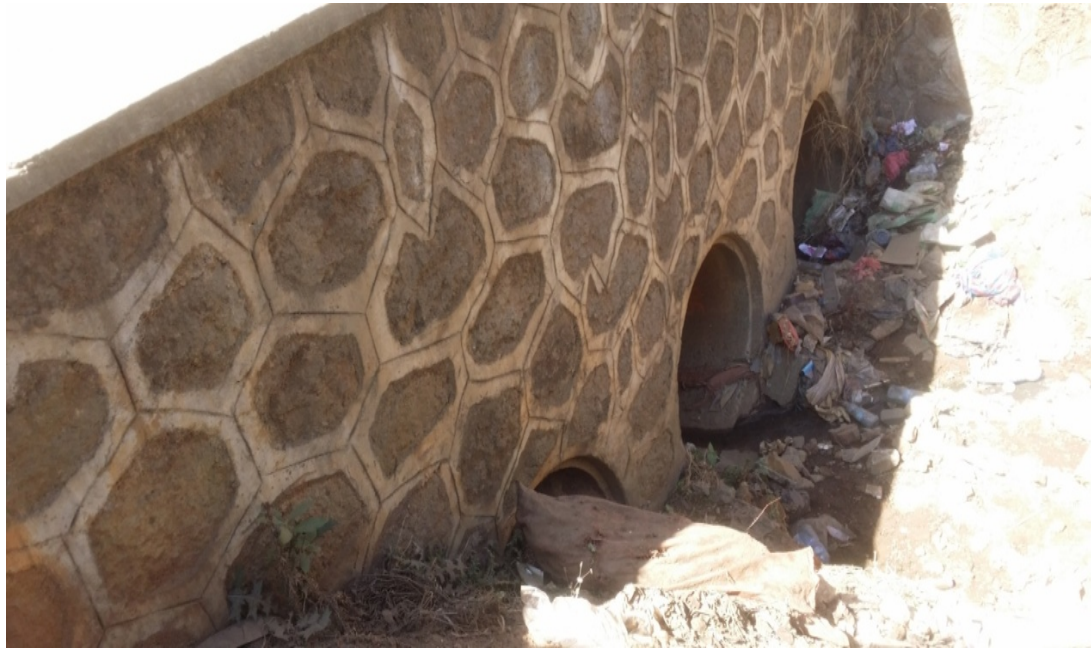
Figure 4.1 Siltation of existing Culvert
