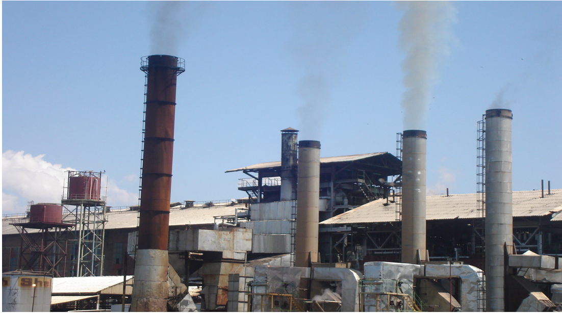
Fig. 3.1 Boilers of MSF
