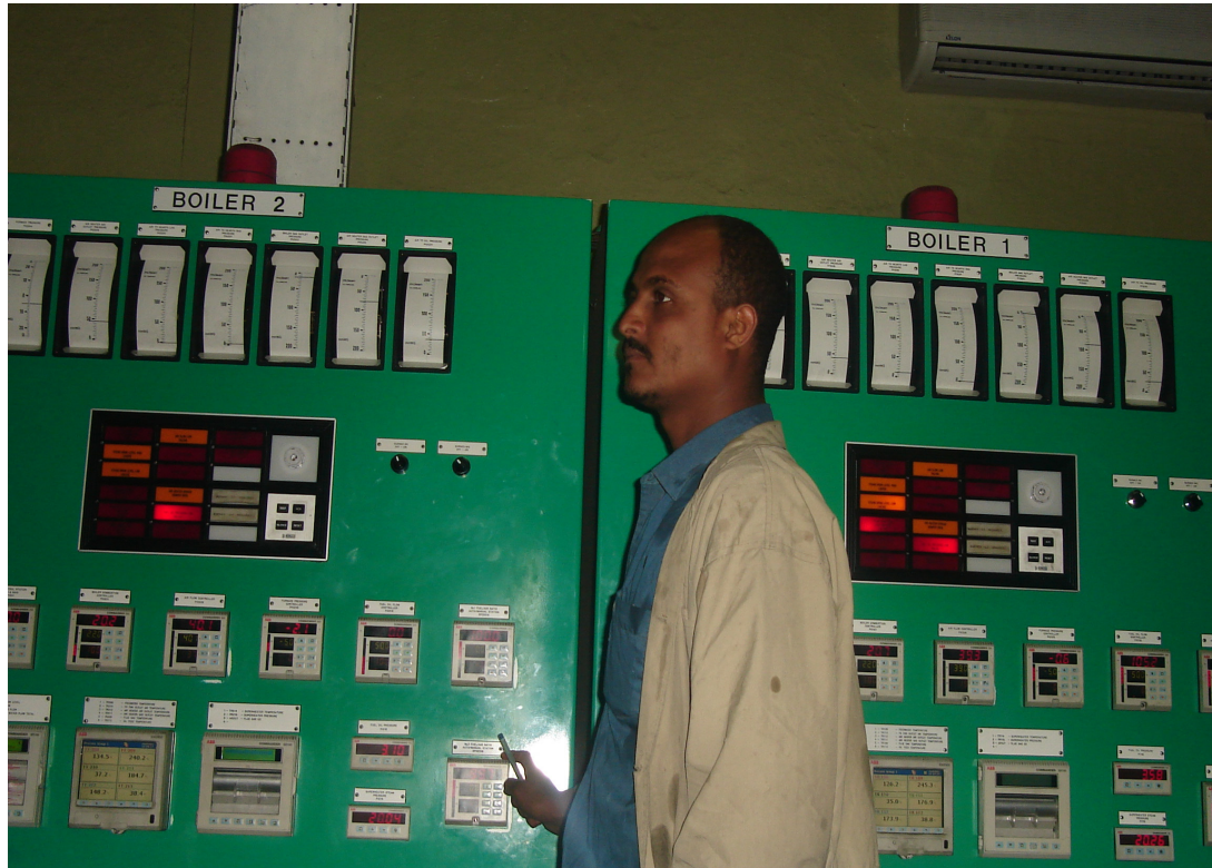
Fig 3.2 Boiler control panel of MSF
