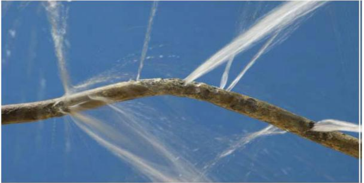
Figure 17: Water Leakage in Addis Ababa
