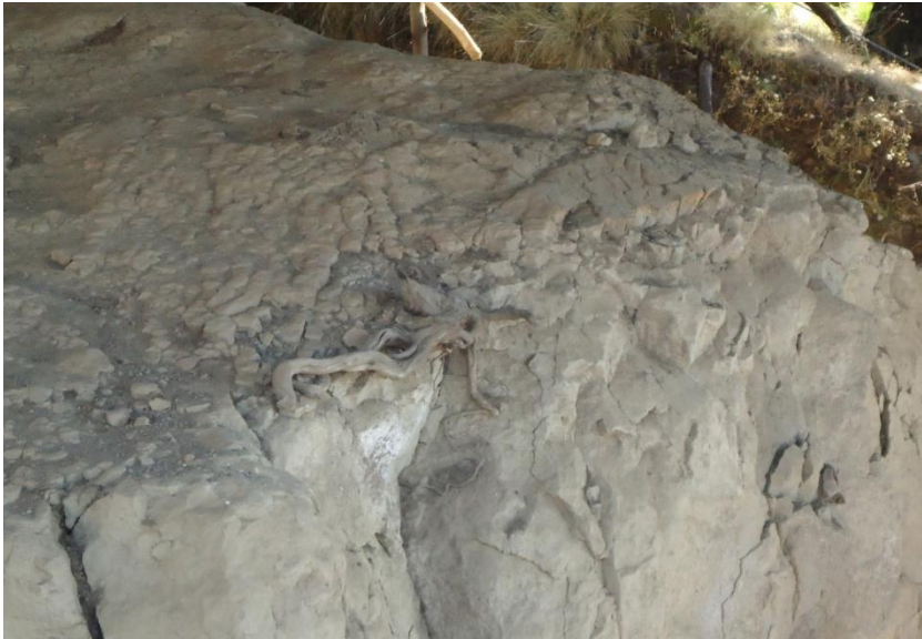
Figure 4. 4: Highly degraded roof of Kenkenit Mikael
