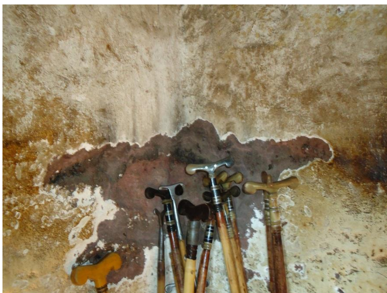
Figure 4. 5: deteriorated plaster; on a column in the church of Genete Maryam
