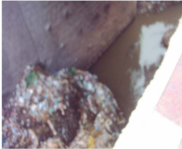
Plate 11: Accumulation of waste in side bridge of river
